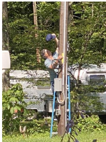
Doug assisting with Wi-Fi restoration following the June power outage
